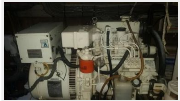
Northern Lights Generator
