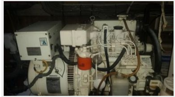
Northern Lights Generator
