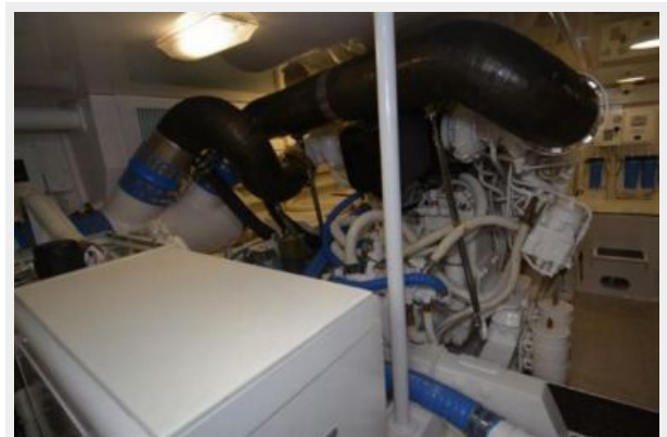
Engine Room Aft Port
