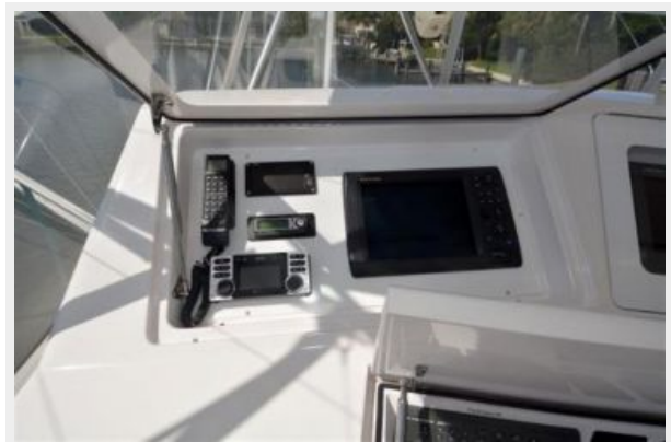
Outboard Electronics Box
