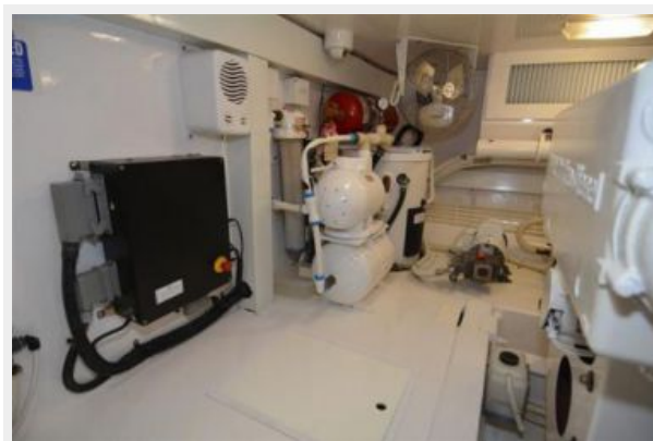
Engine Room Forward Stbd
