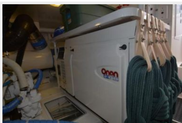
Onan 21.5 KW Generator
