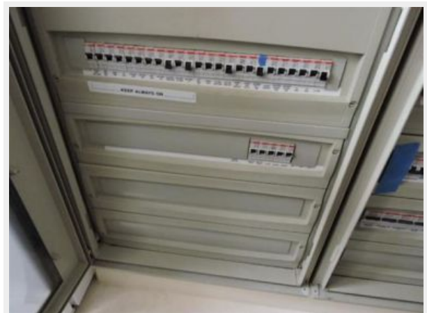
Engine Room Breakers 2
