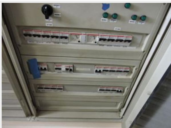
Engine Room Breakers
