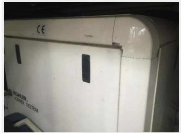
15.5kw Kohler generators
