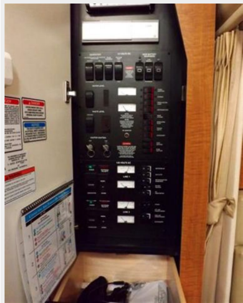
Electrical panel close-up
