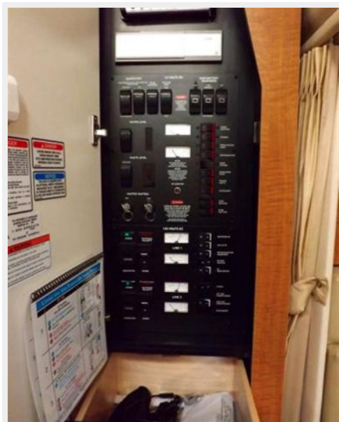
Electrical panel close-up
