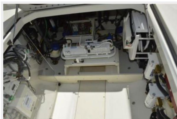
Clean Mechanical Compartment
