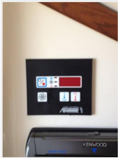
Main Cabin 5 - A/C
