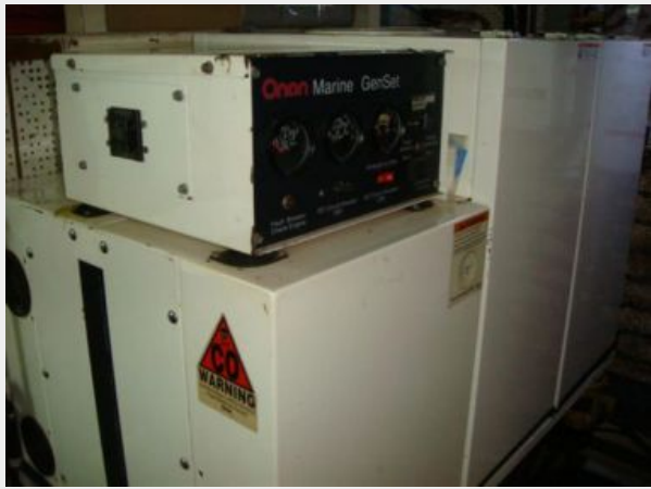
48' Defever Onan Generator Soundbox
