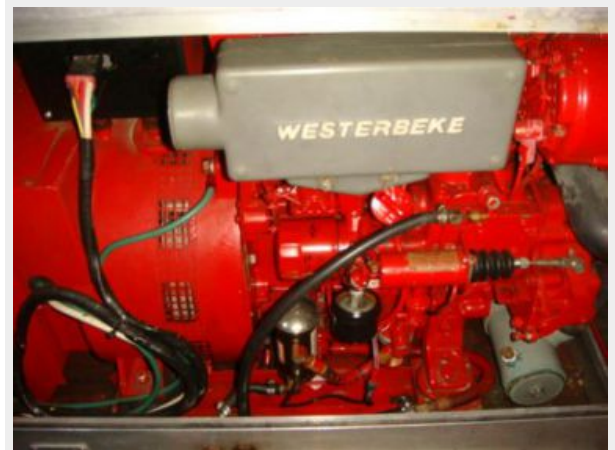
48' Defever Westerbeke Generator
