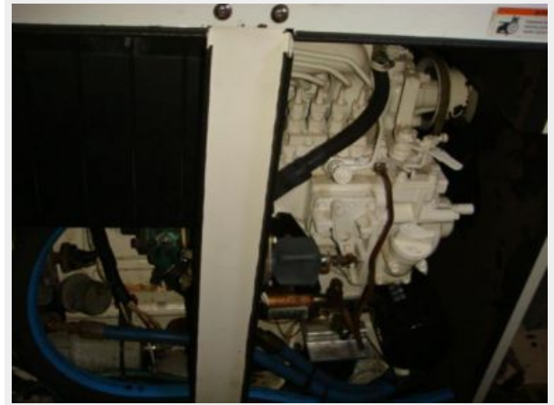
48' Defever Onan Generator
