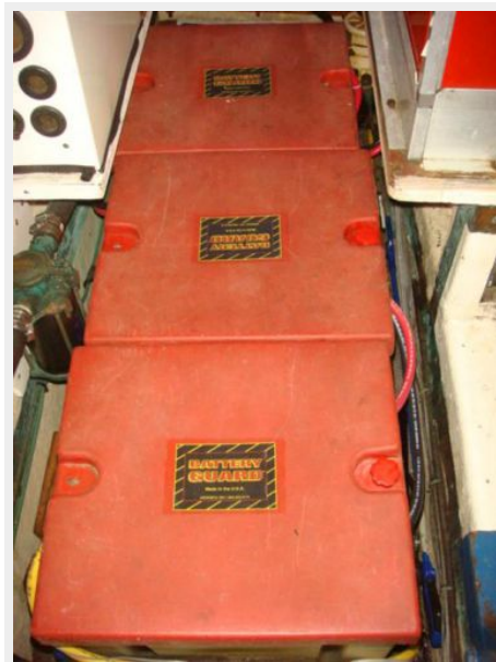
48' Defever Battery Bank
