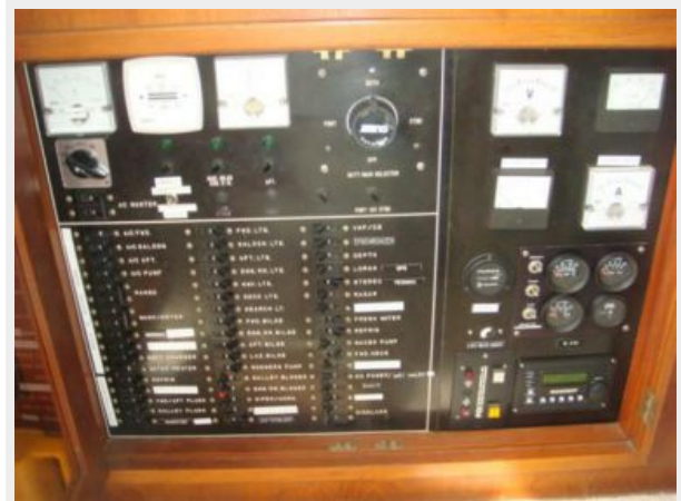
48' Defever Electrical Panel
