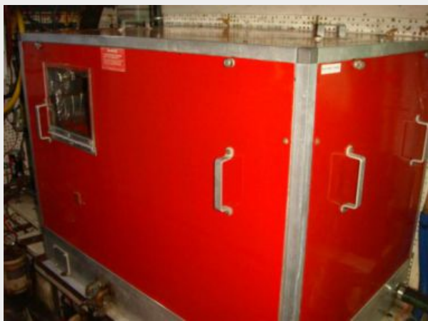
48' Defever Westerbeke Generator Soundbox
