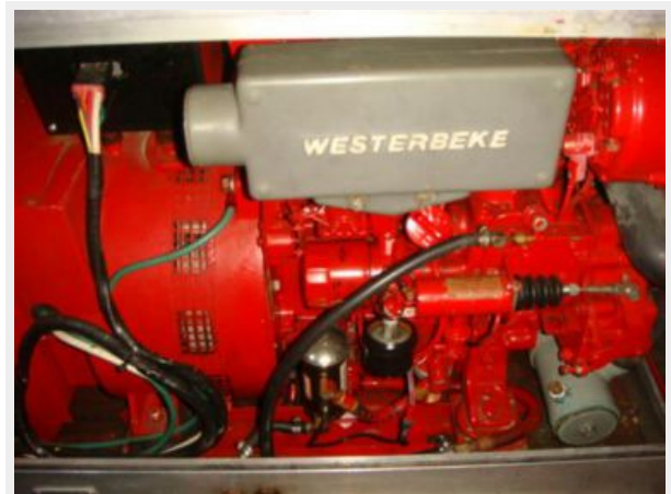
48' Defever Westerbeke Generator
