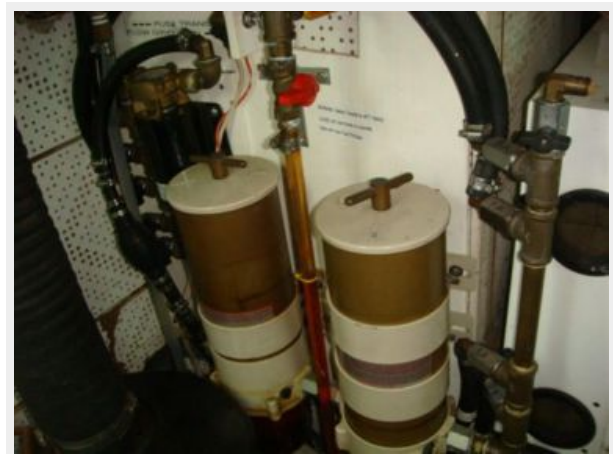
48' Defever Port Racor Fuel Polishing Filters
