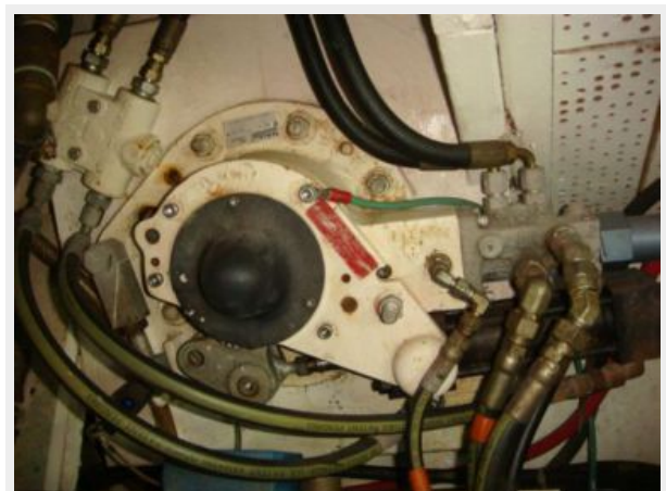
48' Defever Starboard Stabilizer Head
