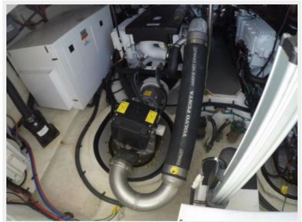
Generator w/sound shield
