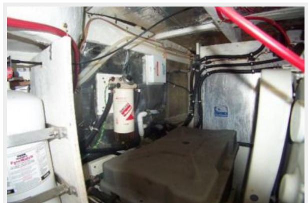
Forward view of Engine Room
