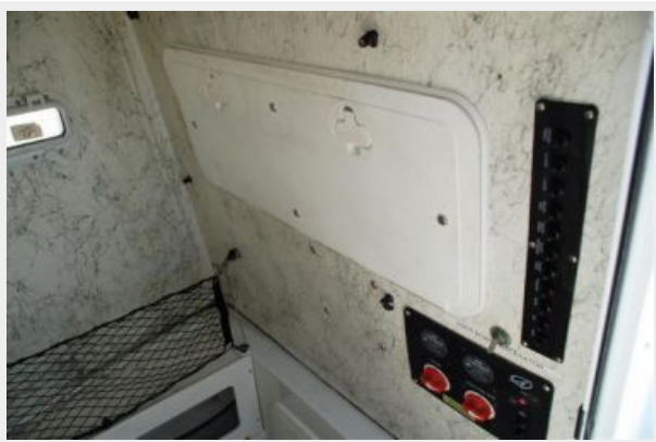
Access to Helm Electronics
