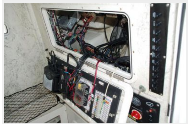
Access to Helm Electronics
