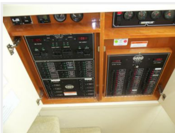
Companionway Electrical Panel
