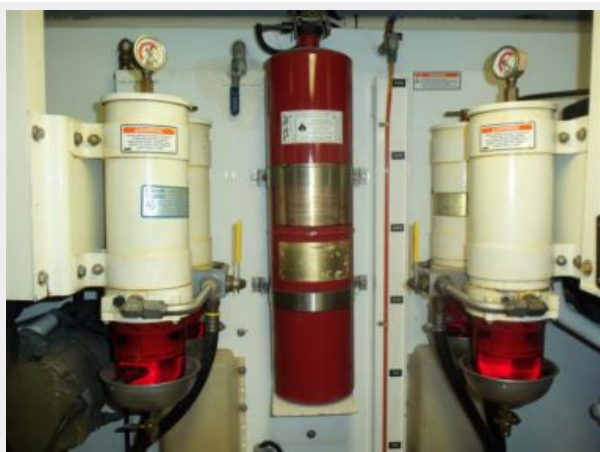
Engine Room Forward
