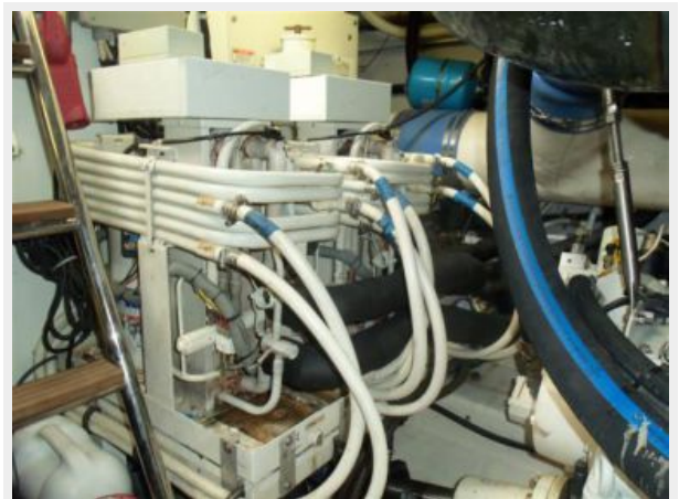
Chilled Water AC
