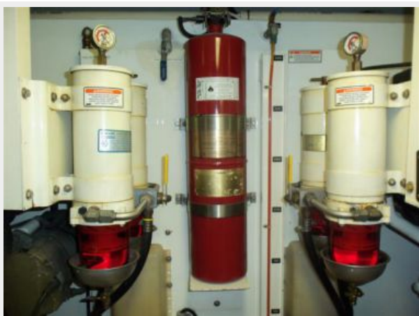
Engine Room Forward
