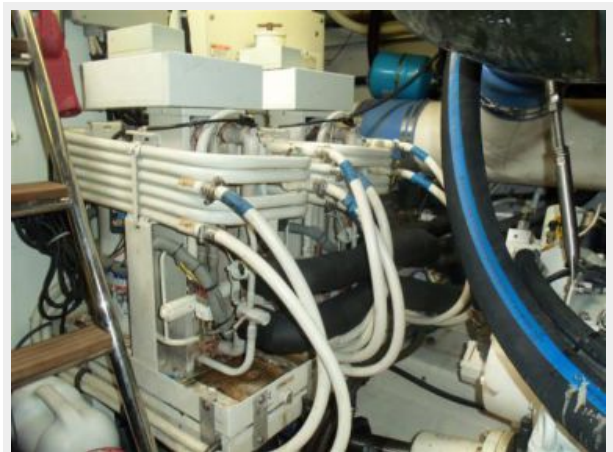
Chilled Water AC
