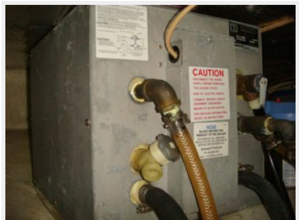
37' Pacific Trawler water heater
