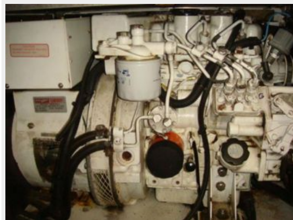
37' Pacific Trawler generator
