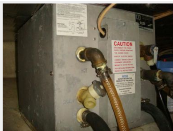
37' Pacific Trawler water heater
