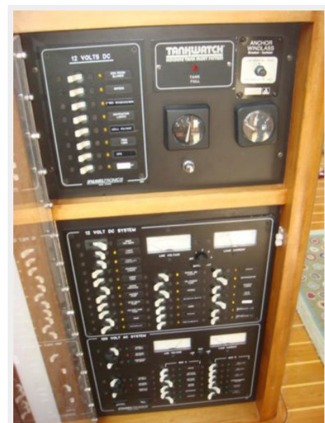
40' Legacy Electrical Panel
