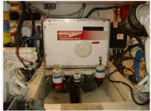
40' Legacy Engine Room Aft
