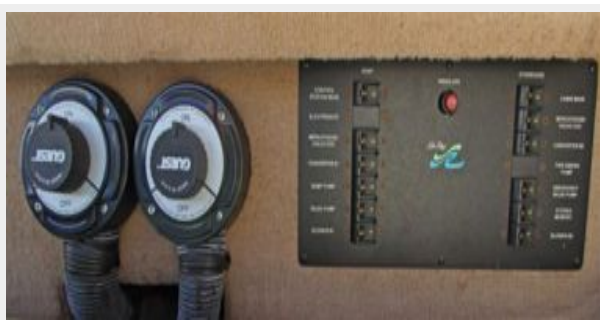
Guest Battery Switches & Main Breaker Panel Located In Cockpit
