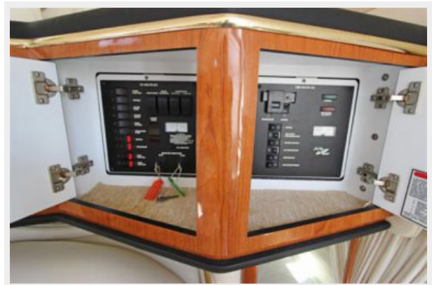
AC/DC Electrical Panel Located In Salon
