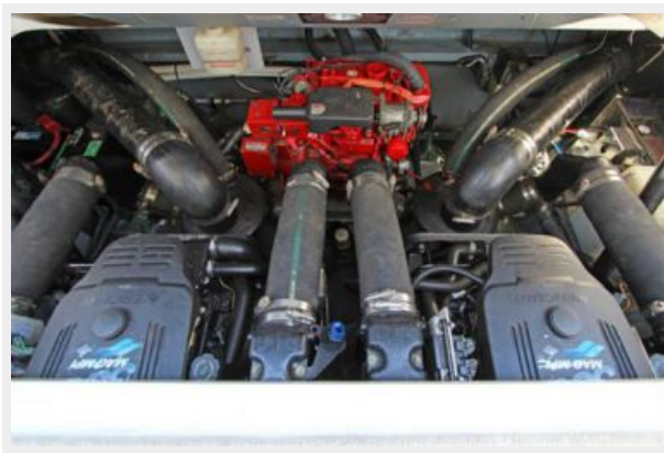
MerCruiser 350 MAG MPI Engines & Westerbeke Generator
