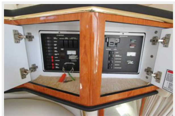
AC/DC Electrical Panel Located In Salon
