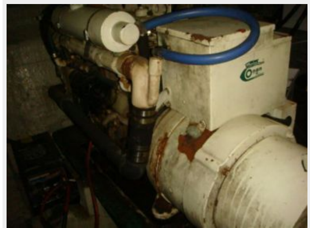
45' Chris Craft Generator photo2
