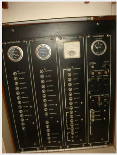
45' Chris Craft Lower Helm Electrical Panel
