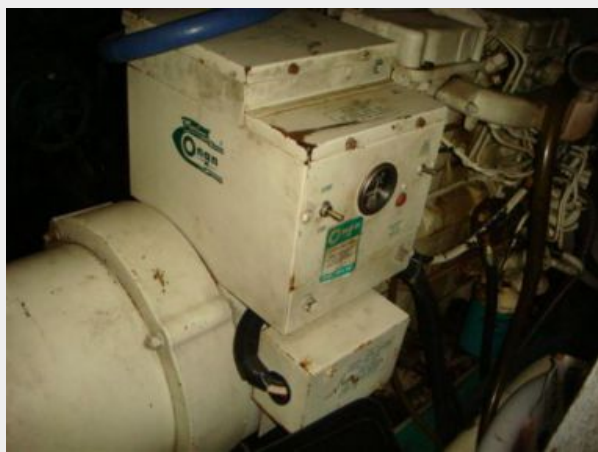
45' Chris Craft Generator photo1
