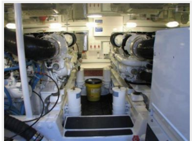
Engine & Mechanical Equipment 1 - Engine Room
