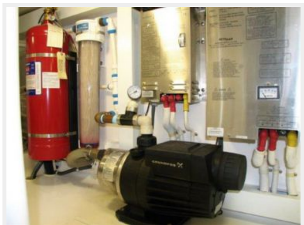
Engine & Mechanical Equipment 7 - Engine Room
