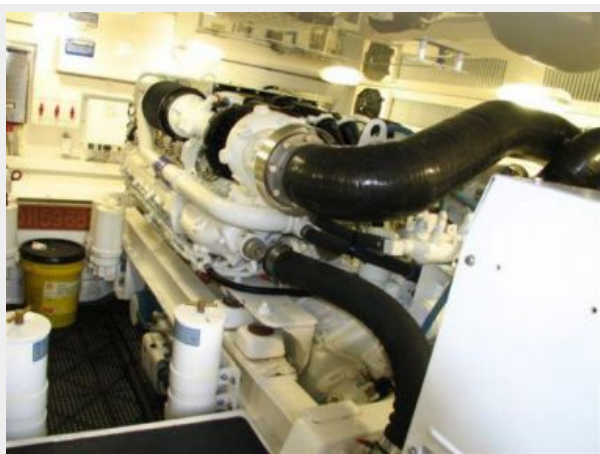
Engine & Mechanical Equipment 4 - Starboard Engine
