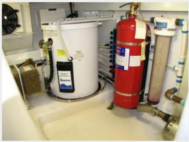
Engine & Mechanical Equipment 8 - Engine Room
