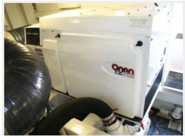
Electrical System / Equipment - Onan Generator
