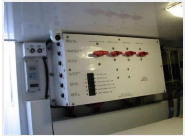
Engine & Mechanical Equipment 9 - Engine Room
