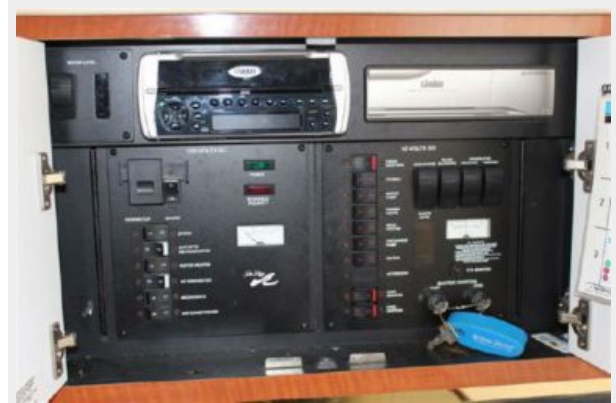
Main Distribution Panel
