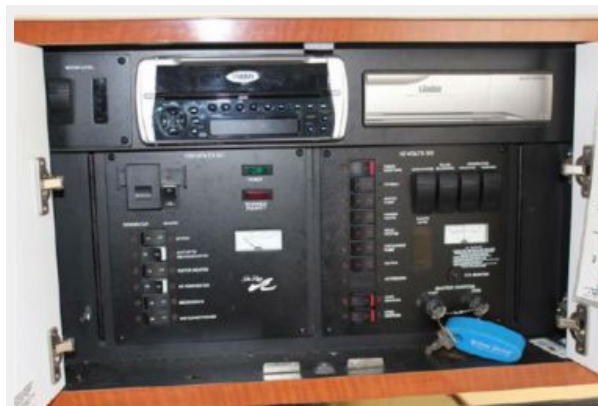
Main Distribution Panel
