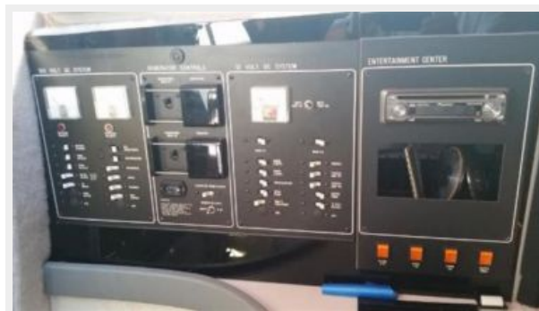
Salon Control Panel
