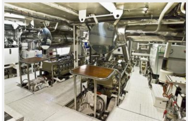
Clean and well maintained engine room with plenty of room!
