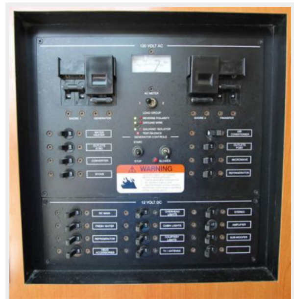
AC/DC Electrical Panel Located In Salon
