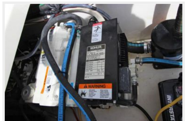
Kohler 5kw Generator W/150 Hours (Full Service June 2015)
