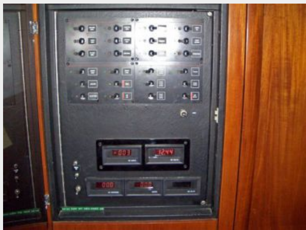
AC Service Panel
