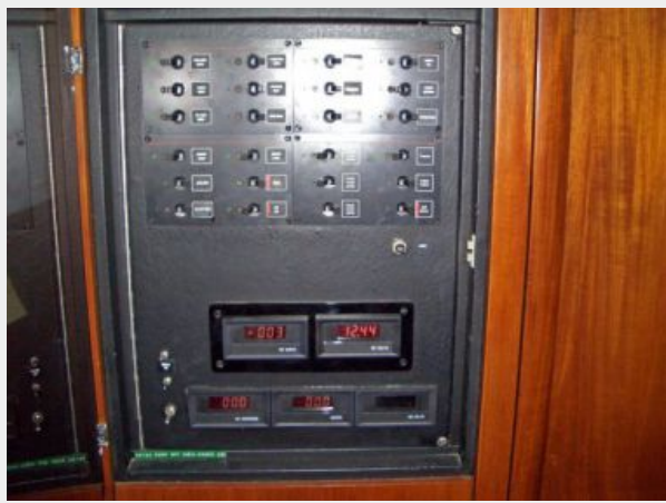
AC Service Panel
