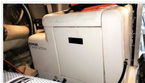
50' Navigator Kohler Generator
