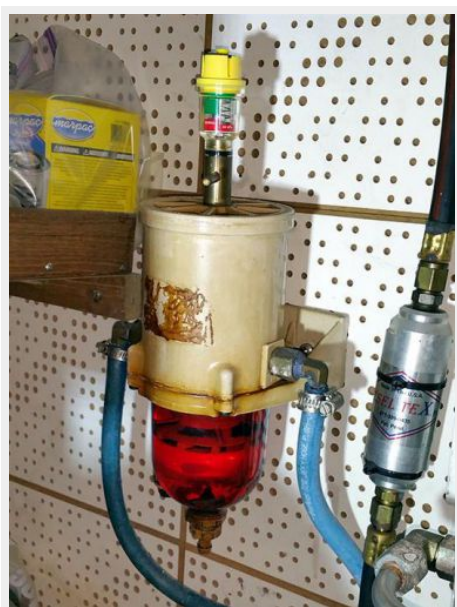
40' Albin Genset Racor Fuel Filter
