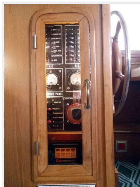
40' Albin Electrical Panel
