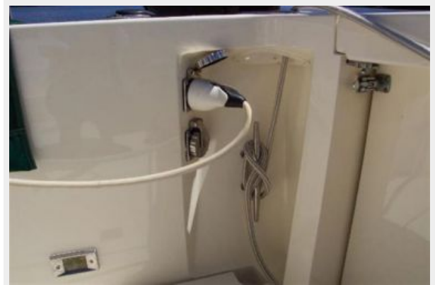
Dockside Electrical Connection
