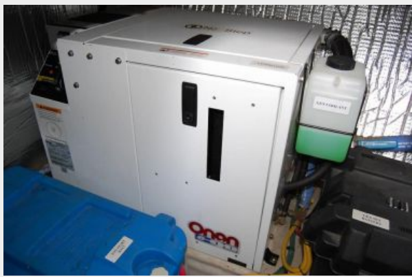
Engine Room Generator
