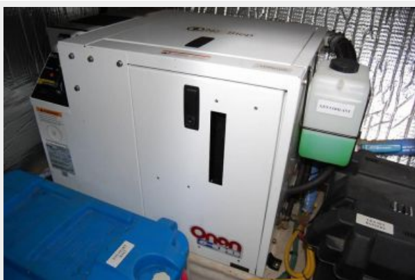
Engine Room Generator
