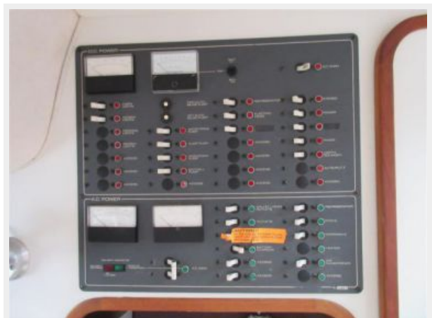
31' Tiara Electrical Panel
