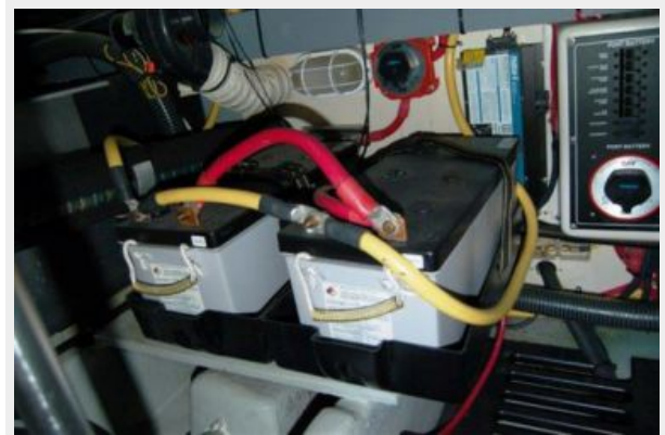
Electrical Battery Banks
