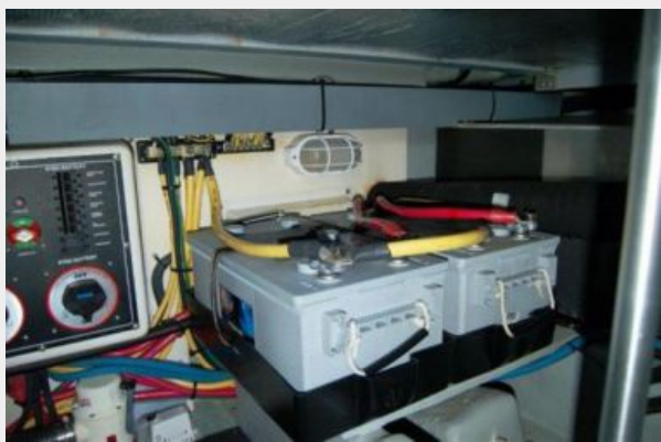
Electrical Battery Banks
