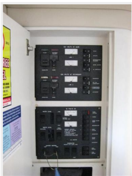
AC/DC Electrical Panels
