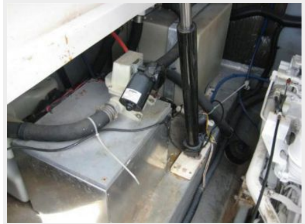
Water Heater & Holding Tank
