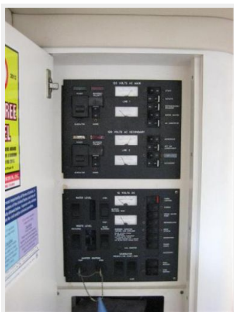
AC/DC Electrical Panels
