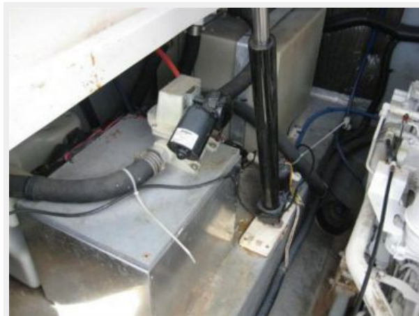
Water Heater & Holding Tank
