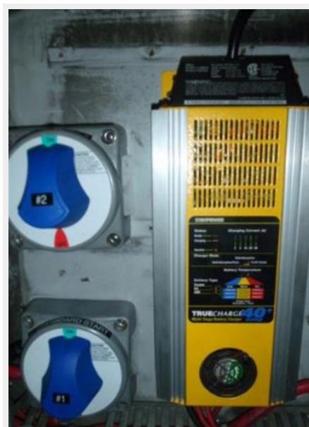
Battery Charger with Select Switches
