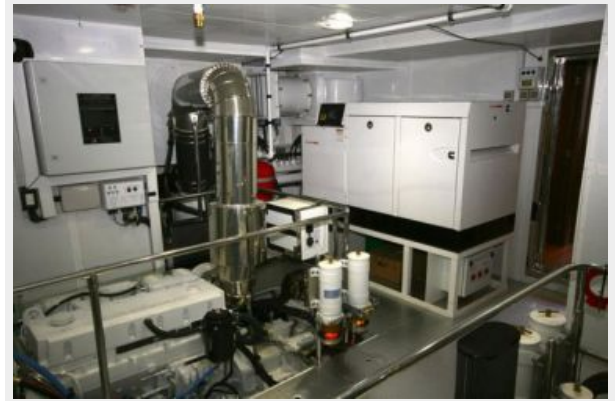
Engine Room - looking aft
