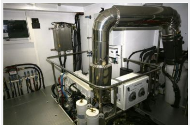
Engine Room - looking to starboard
