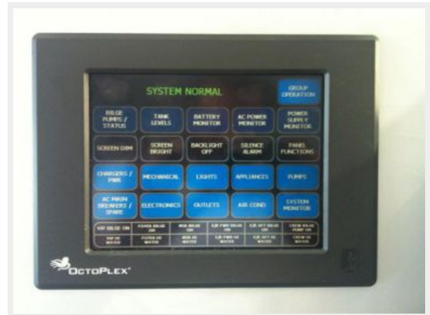
Octoplex control panel
