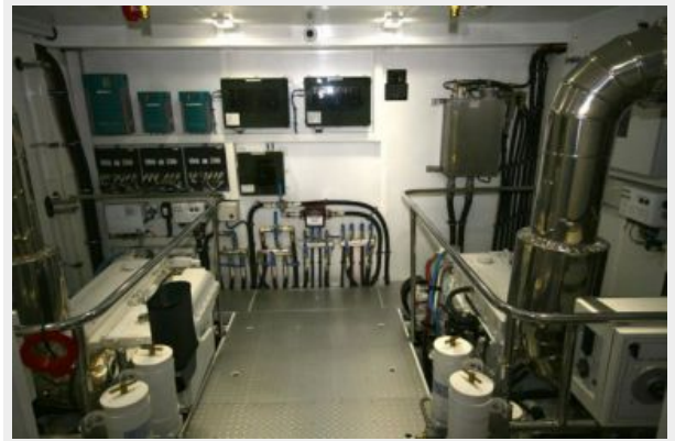
Engine Room - looking forward
