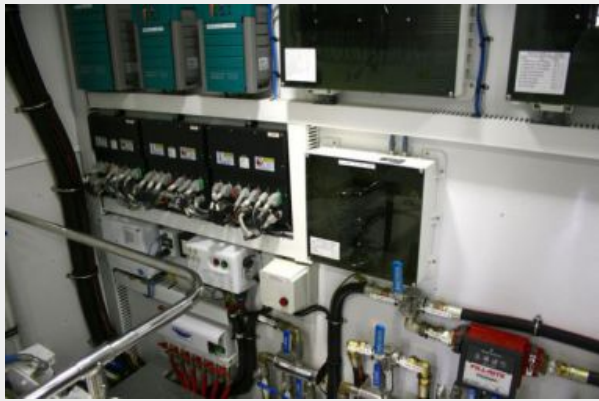
Engine Room - detail
