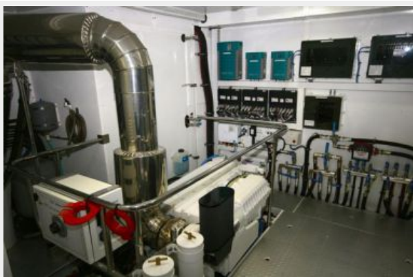
Engine Room - looking to port
