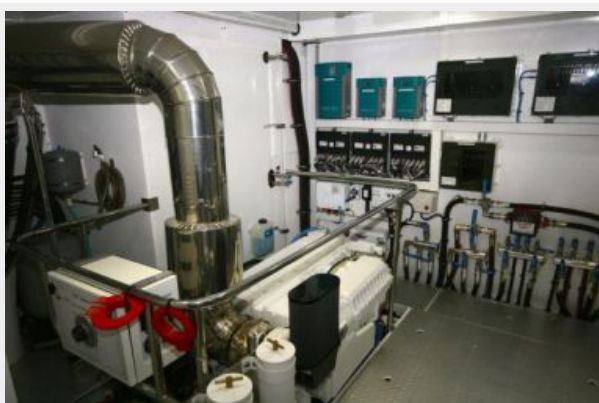
Engine Room - looking to port
