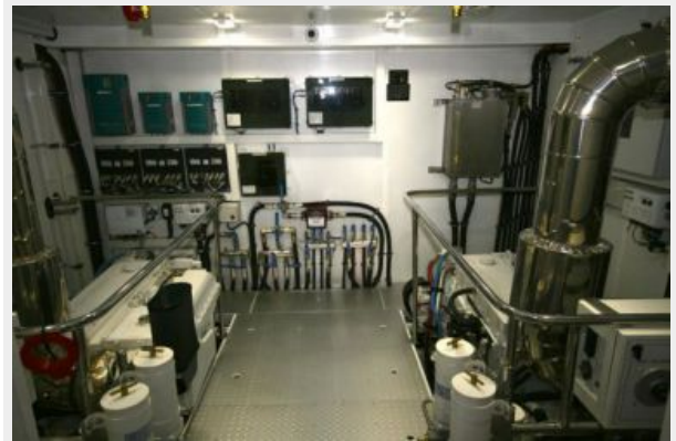
Engine Room - looking forward
