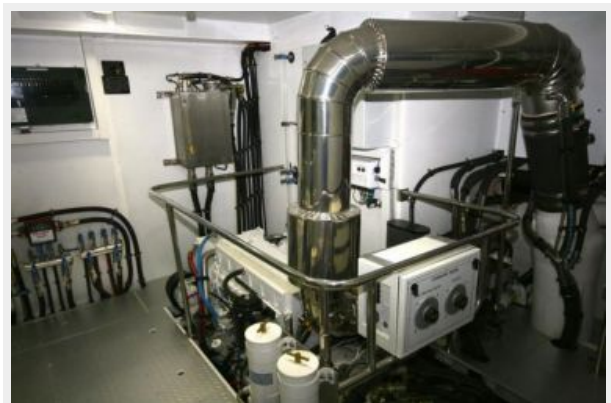
Engine Room - looking to starboard
