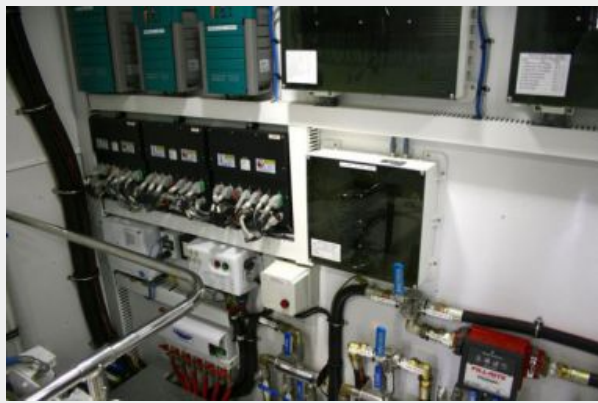
Engine Room - detail
