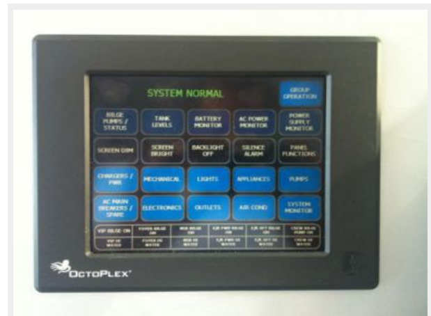
Octoplex control panel
