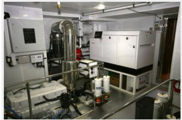
Engine Room - looking aft
