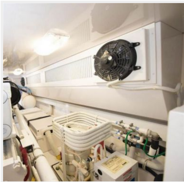
Engine Room Port Outboard
