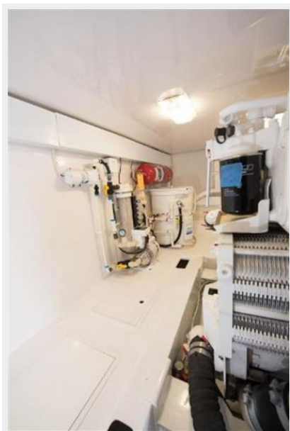
ENgine Room Starboard
