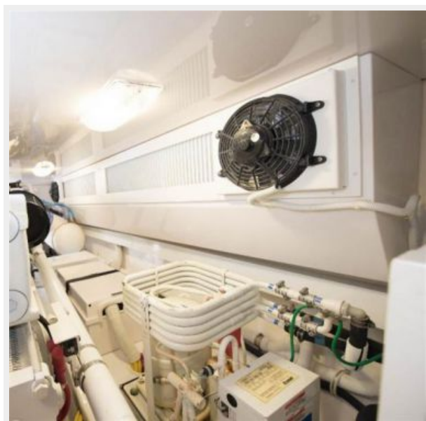
Engine Room Port Outboard
