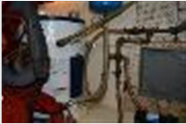
Engine room with new water heater
