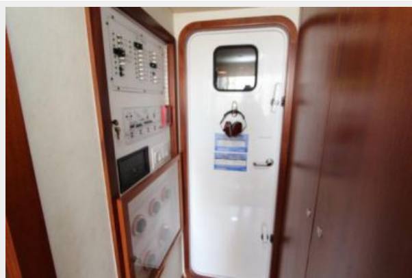
Control panel / Watertight door to engine room
