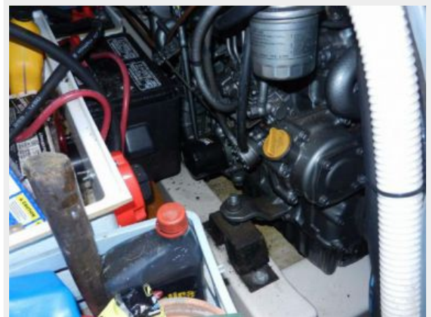
Good access panels
