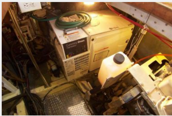
ONAN Genset with sound enclosure
