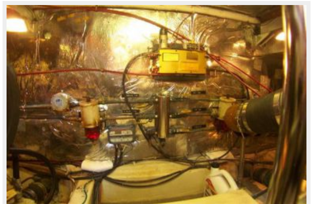
Engine Room - aft
